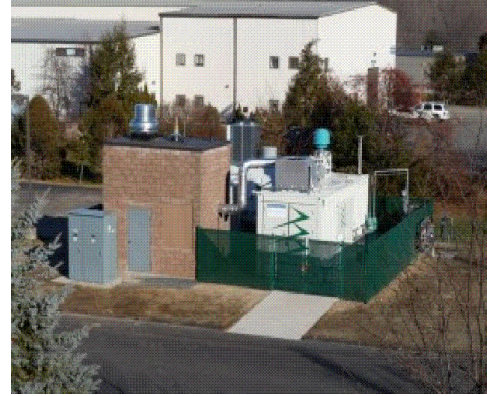
Figure 1. 300 kW e DFC fuel cell power plant.
