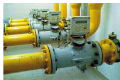
Figure 2. Basement Equipment Room.
